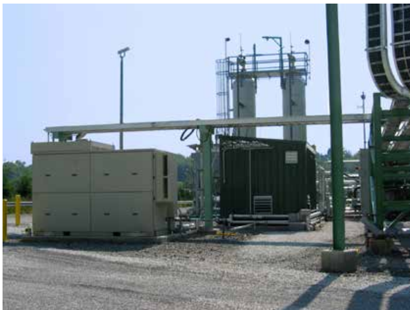
Capstone CR200 microturbine integrated with the Fallowfield Gas Processing Plant.
