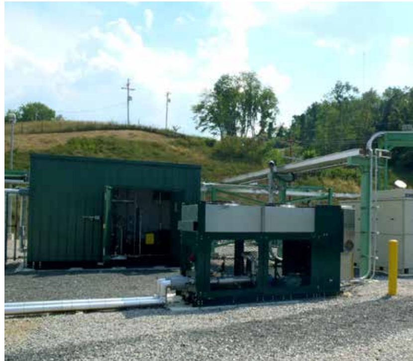
The microturbine system includes a gas conditioning skid, chiller, and microturbine.
