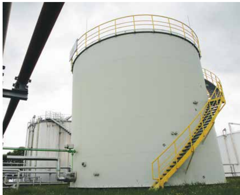
A Capstone C65 microturbine produces electricity for the facility and may use heat exhaust and warm facility buildings for process heating, and to heat pipelines.
